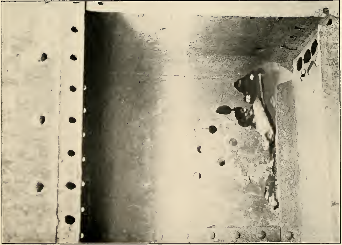
Effect of Acid upon lower corner of steel lock gate, Lock No. 2, Monongahela River, thickness of plate \frac{1}{2} inch.
